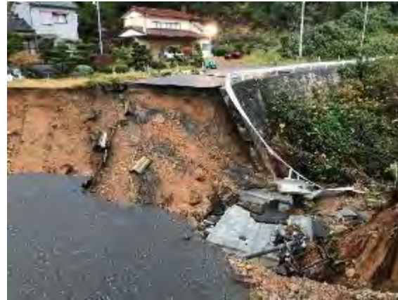
Collapse of a city road on the Shigemo Peninsula, isolated village Helicopter transport of supplies
