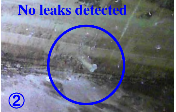
San cushion drain pipe end
