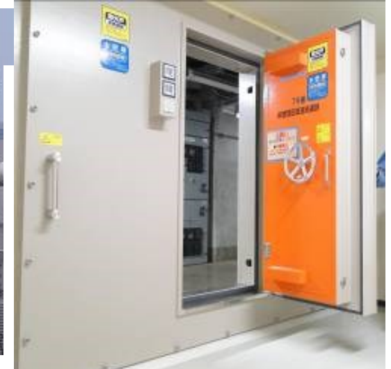
Water-tight door : Preventing flooding of critical areas (~60 places)
