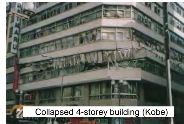
Damage to Port of Kobe
