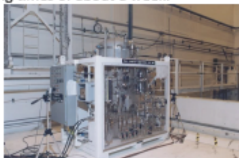
Canister Dewatering Machine in the Pool Area
