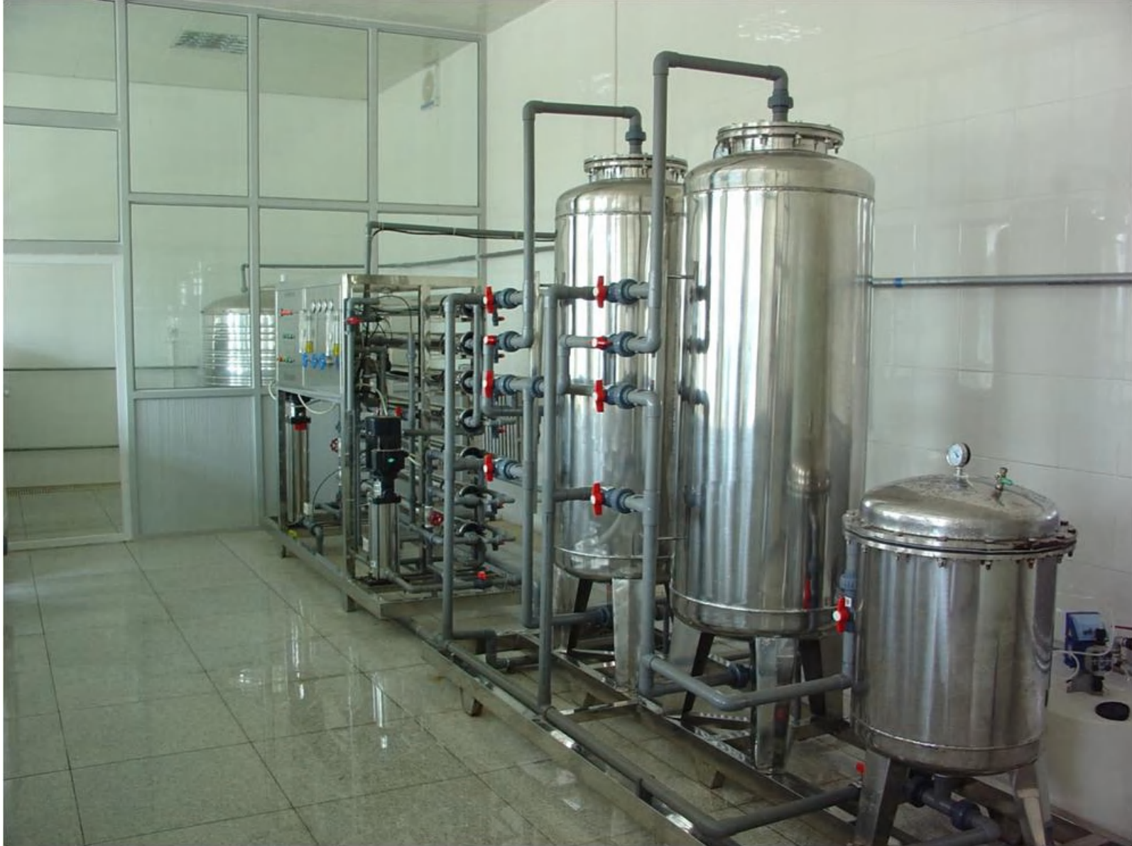
Groundwater treatment plant in Tianjin
