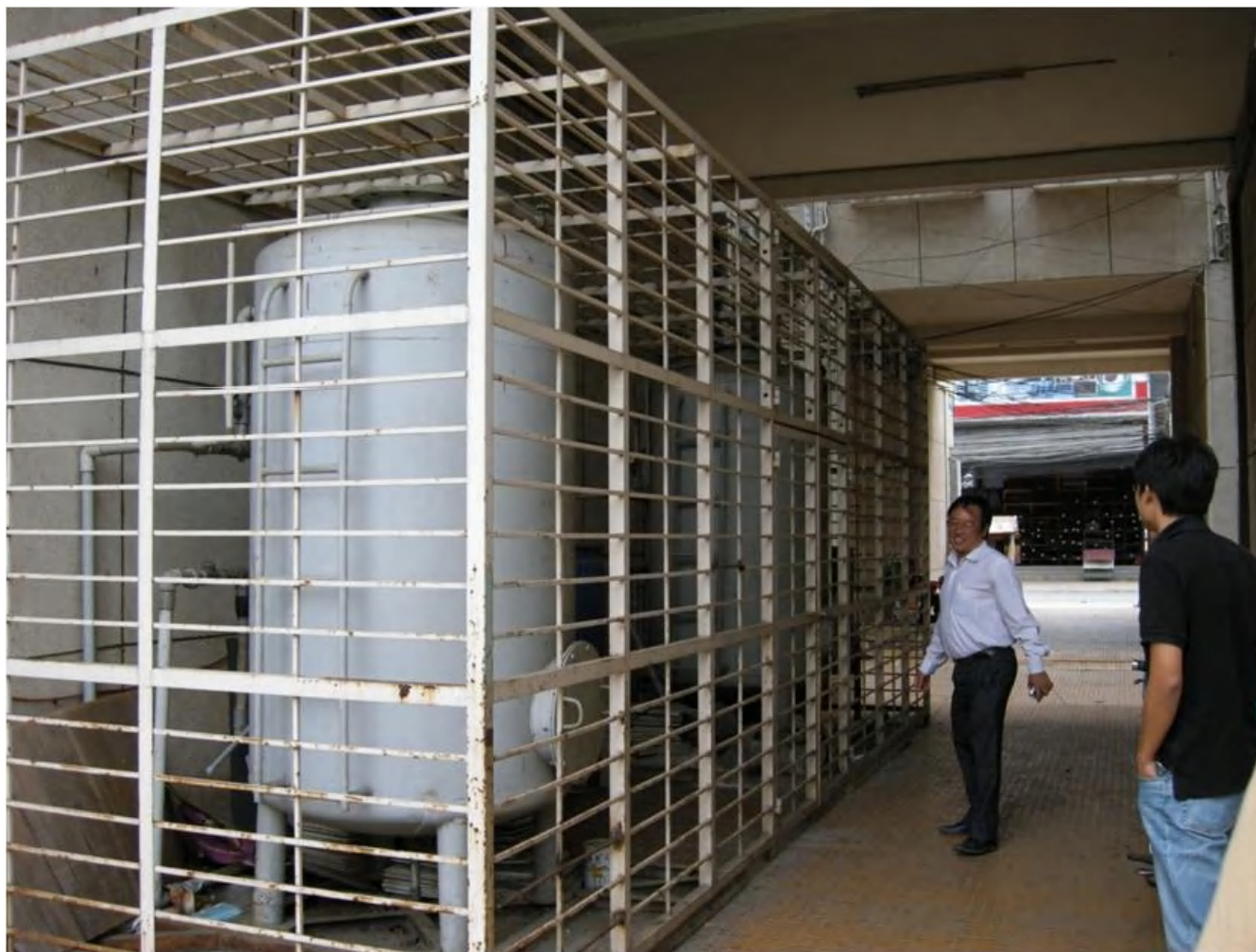
Sand Filtration of Community Groundwater Supply System (Ho Chi Minh City)
